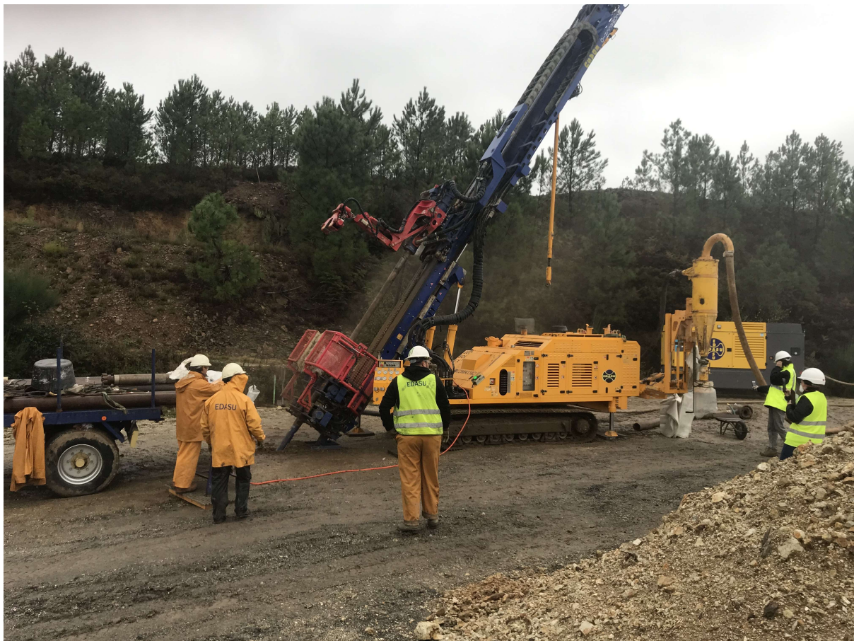
Figure 1: EDASU S.L’s Reverse Circulation rig drilling the first hole in the 2023/24 drilling programme
